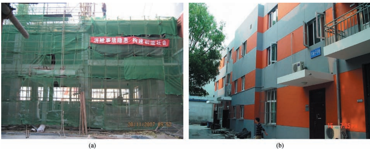
Fig. 19 No. 6 building in Beijing University of Civil Engineering and Architecture. (a) Construction of No. 6 building with RAC in Beijing, China; (b) completed No. 6 building with RAC in Beijing, China
