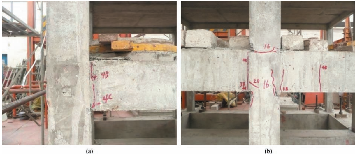
Fig. 3 Failure pattern of the cast-in situ RAC frame structure. (a) Beam; (b) column
