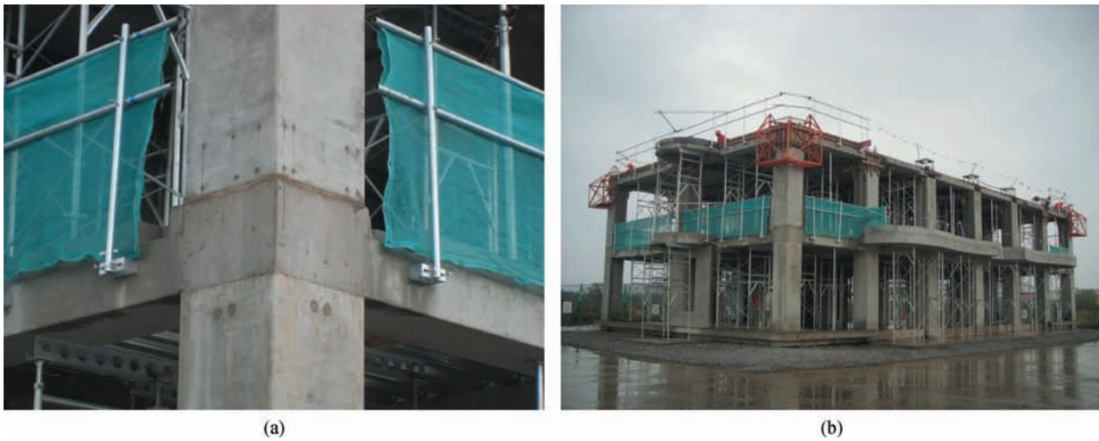
Fig. 17 Shanghai Urban Construction test building half made of RAC. (a) Cast-in situ RAC joint of this building; (b) Shanghai Urban Construction No. 2 building in construction process
