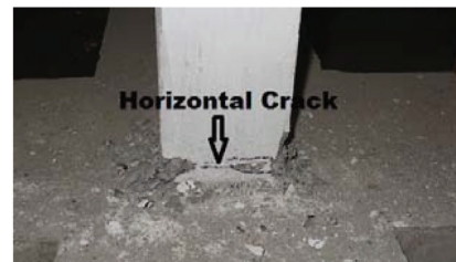
(b) Cracks on the RAC column base
